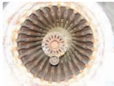
FIGURE 4. A burner in a thermal oxidizer in a sulfur recovery unit combusts the incinerator gas to form SO 2
